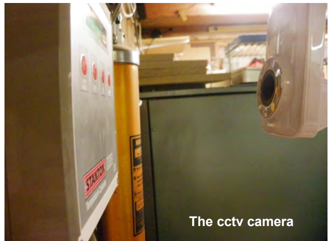
The cctv camera aimed at the kiln’s controller
